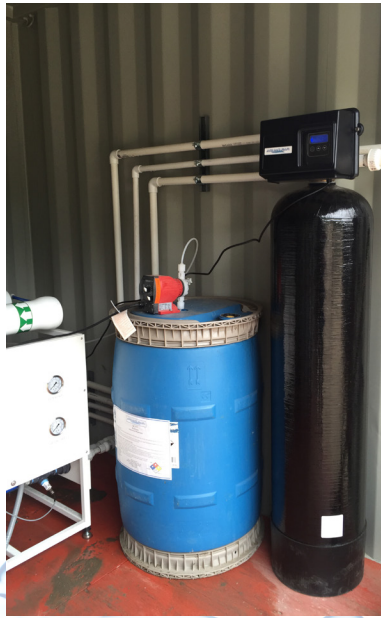
Filtration and antiscalant chemical
