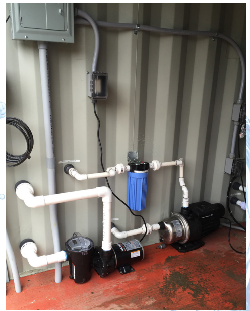
Distribution pumps and calcite filter
