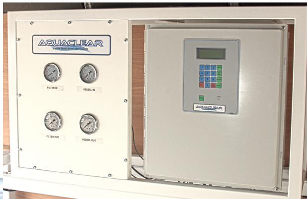
> Local Control Panel
